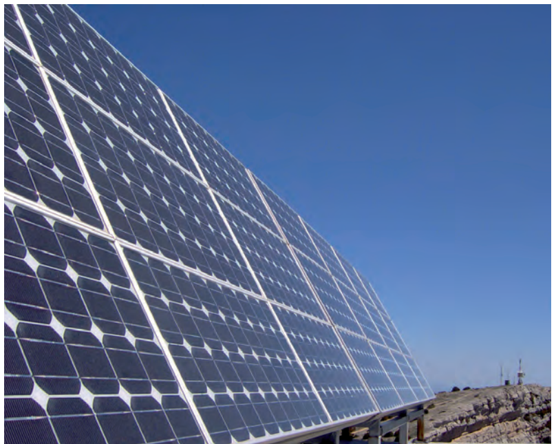
Paneles solares/ Solar panels.
